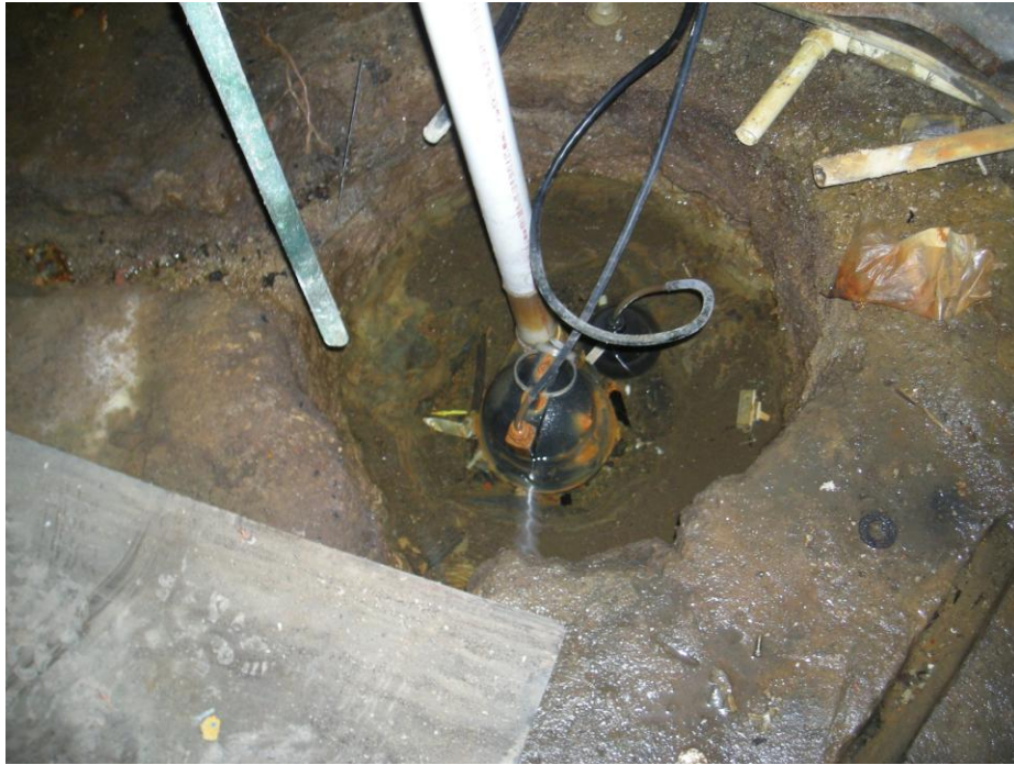
Sump pump is operational
